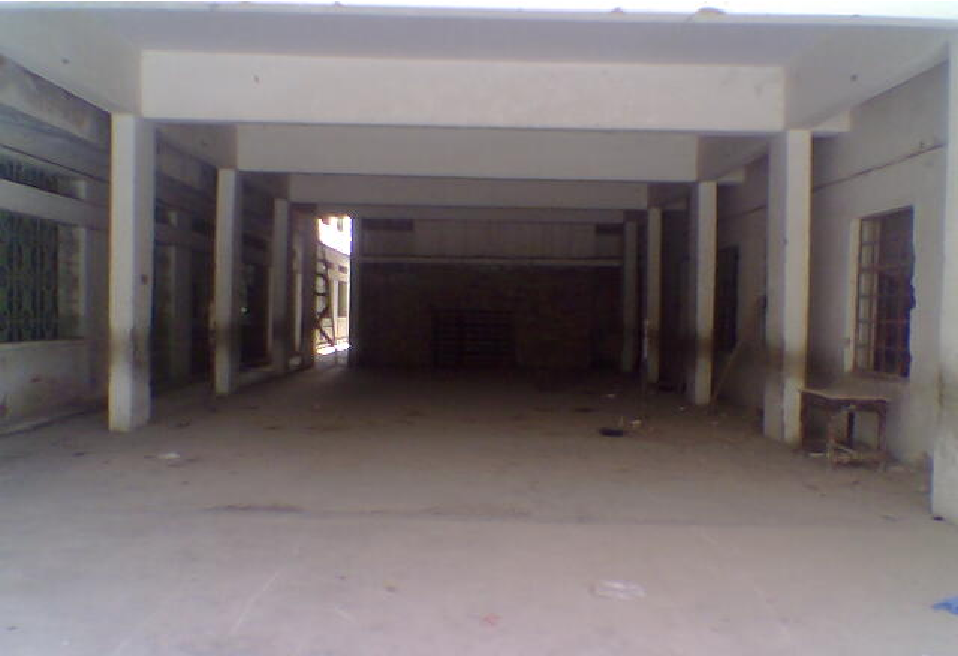
Empty and Dirty Area (Before)
